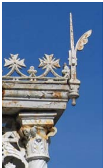
Cast iron finials can be fractured leading to the partial loss of decorative elements
