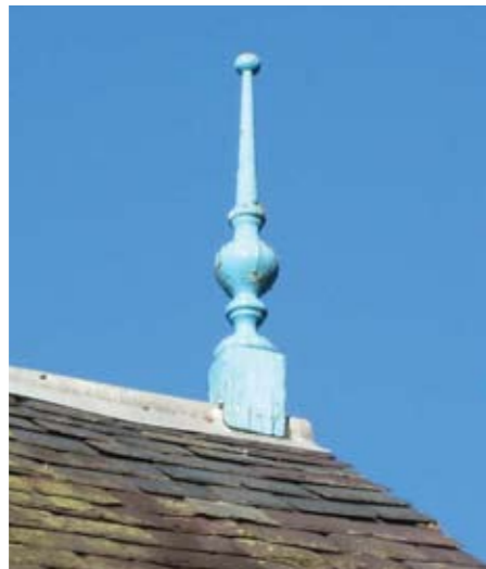
A timber finial in need of maintenance
